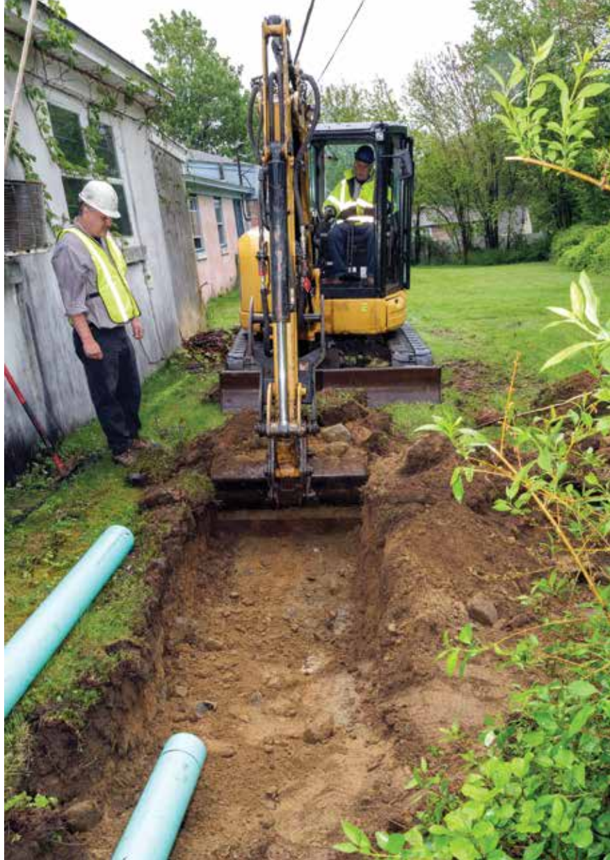
Rees looks on as Peter Orsini excavates a trench in order to lay new sewer pipe.
