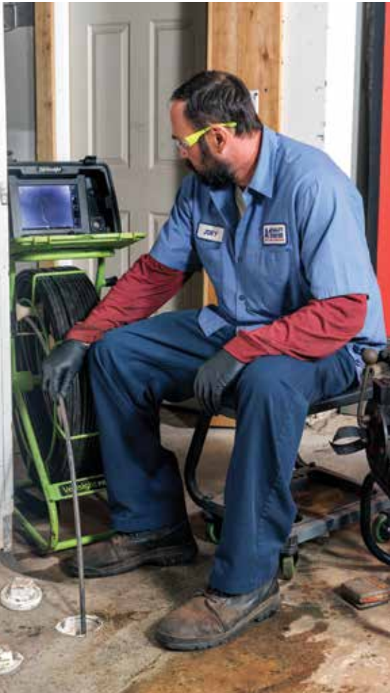
Joey Ryzoc uses an EnviroSight push camera to inspect a sewer line.
